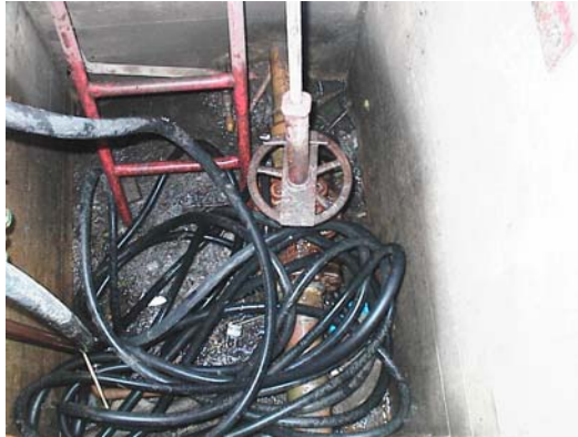
0411WP_PM07 Leaking valve in supply valve chamber
