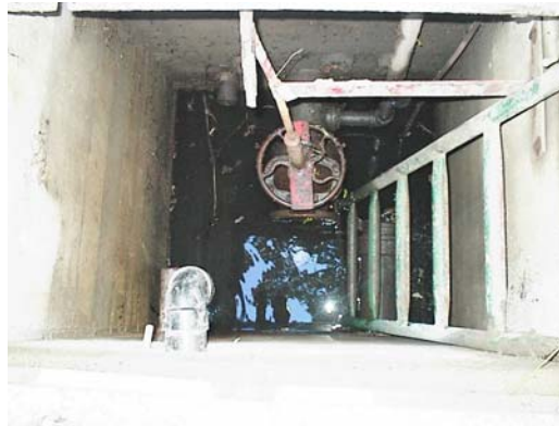
0411WP_PM05 Sump with drain valve
