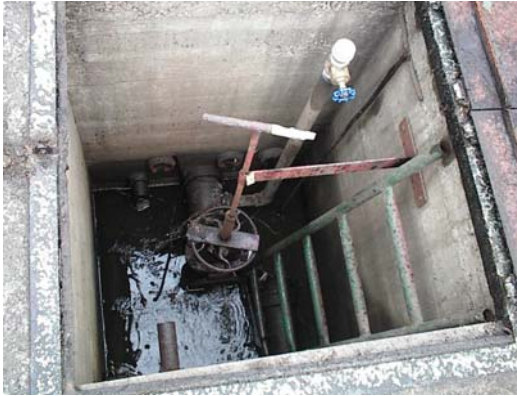
0411WP_PM01 Underground sump with water drain, drain valve and drain to sewer.
