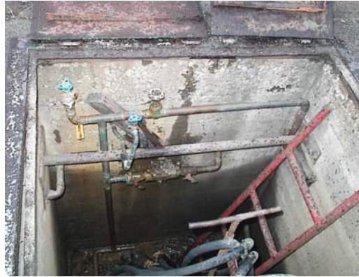
0411WP_PM02 supply valve chamber (underground) with water supply to pool and drinking fountain and fill valve.
