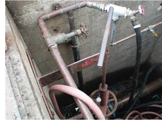
0411WP_PM03 supply valve chamber (underground)
