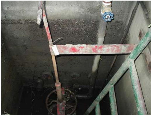
0411WP_PM04 Sump with drain valve
