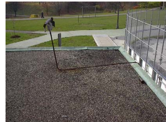
S11-003-R-Bellwoods Exposed/deteriorated membrane at the corner of the roof. Also, sensor on the corner on the roof is not supported.
