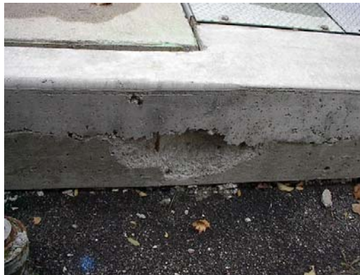
S11-005-R-Bellwoods Pop out concrete at the joint between old and new concrete at the side of the newly installed trench.
