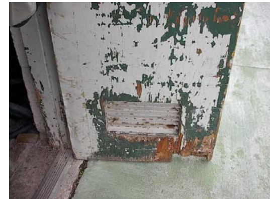
S11-006-R-Bellwoods Rotten wood at the entrance door to the mechanical room.
