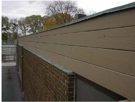
S45-005-R-CampbellPk Through wall flashing between the brick and the wood is copper and very old and damaged.
