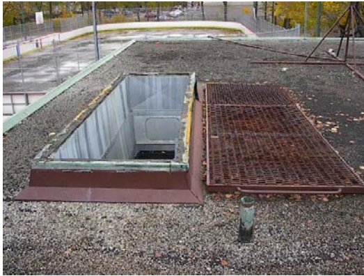
S45-004-R-CampbellPk Exhaust curb on the roof is too low and cover is not installed.
