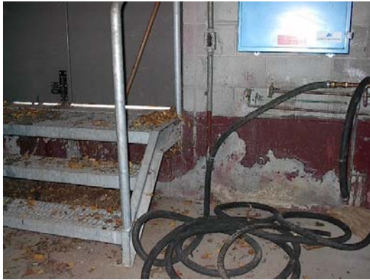
S45-009-R-CampbellPk Bottom of the door does not have any weather proofing and as a result, moisture comes to the inside and wetting the concrete foundation wall, note paint is peeling.
