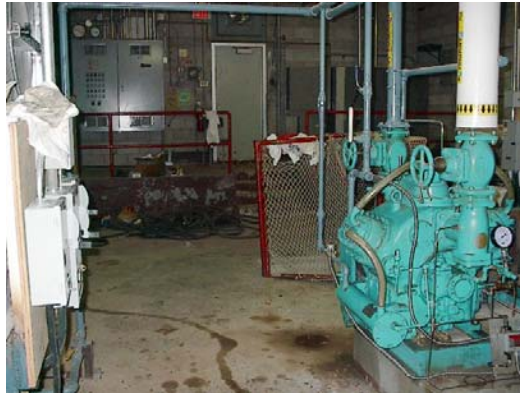
S45-008-R-CampbellPk View of the mech. room, Note that nets are being stored inside the room.
