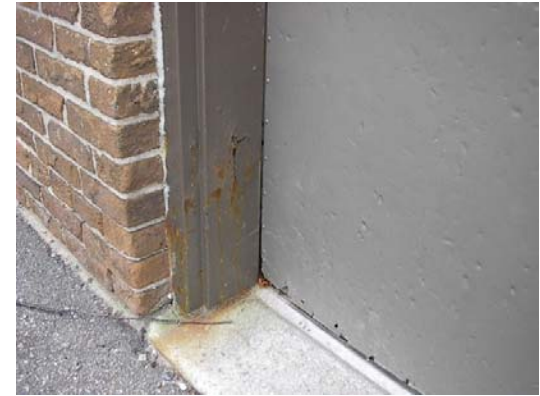
S45-006-R-CampbellPk Bends in the copper have left the top of the brick wall exposed.
