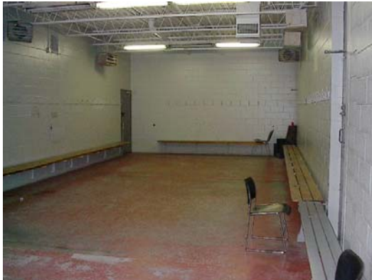
S45-007-R-CampbellPk Corroded metal frame of the exterior doors typical. View of the interior.
